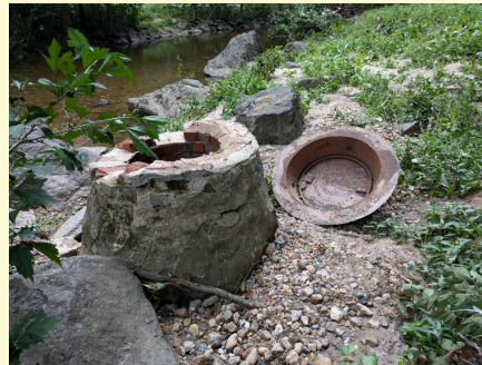
Flood-related damage a parkgoer sent to FOSC. We reported it to WSSC.
