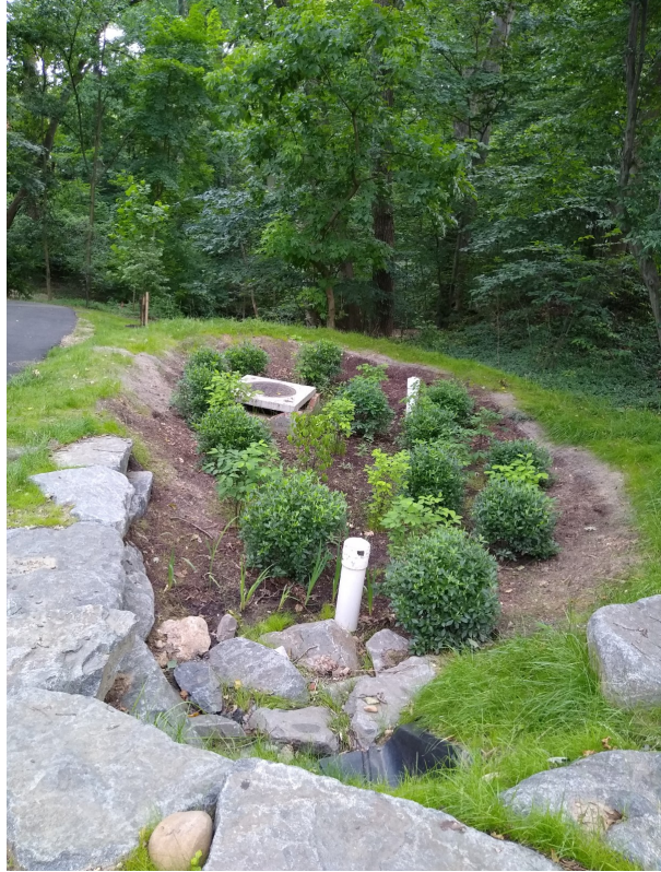
This new rain garden at Merwood collects storm water and allows it to infiltrate slowly and get absorbed by plants.
