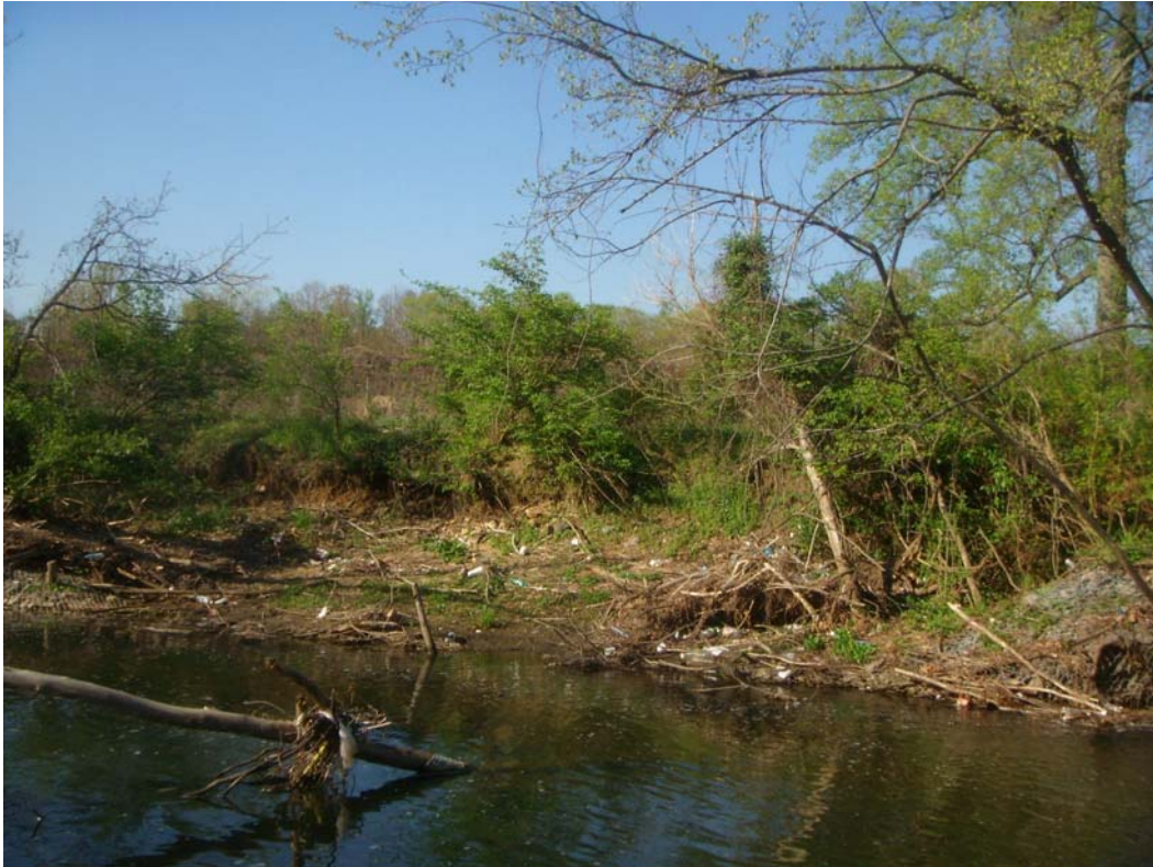
Northwest Branch – 5 Collapsed gabion and bank, April 2008
