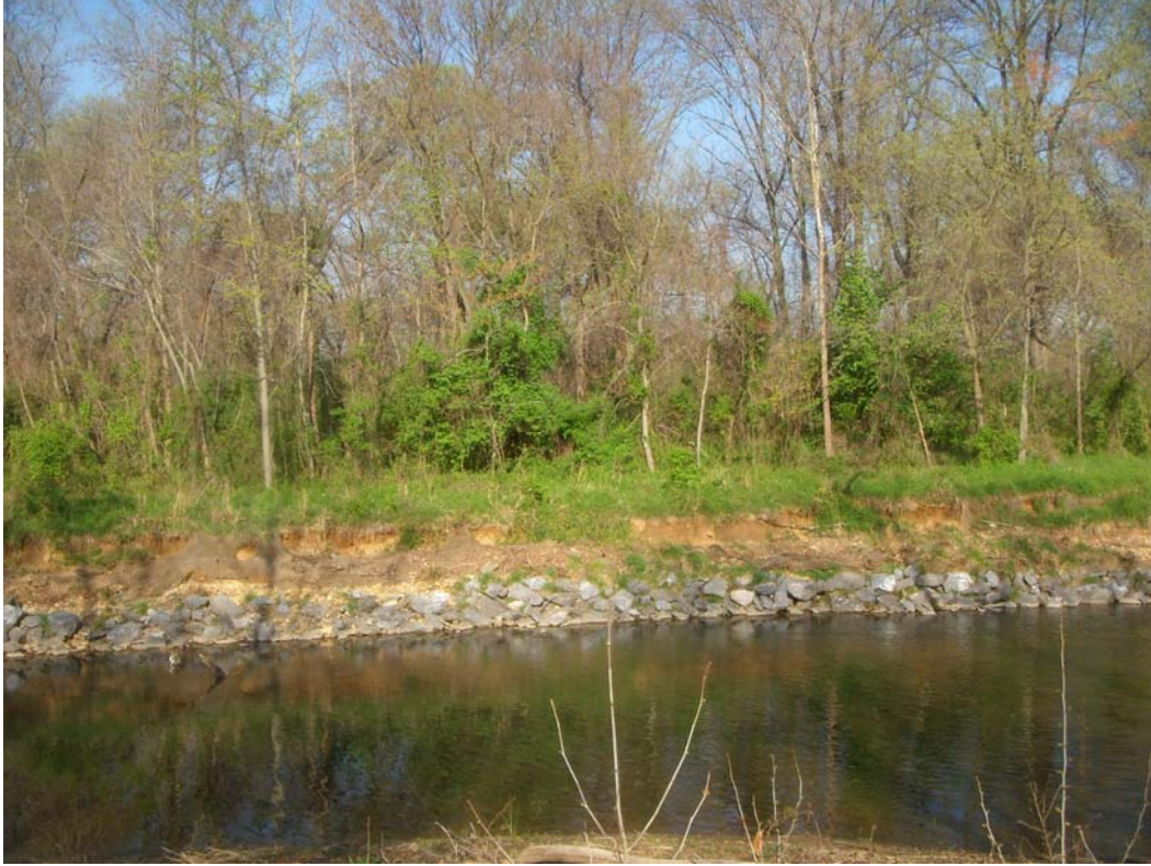
Northwest Branch – 6, erosion on right bank, April 2008
